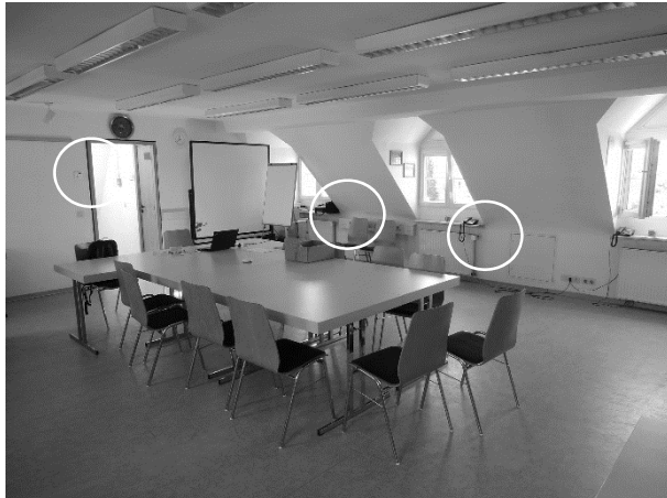
Meeting room: 6 valve actuators, 1 room sensor
