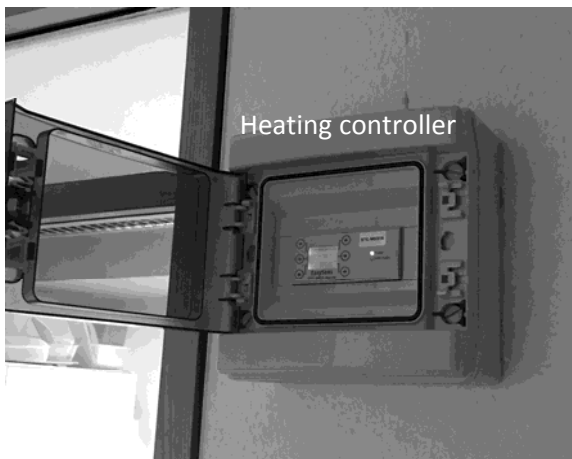
Heating controller (Attic)
